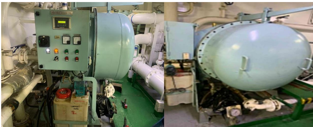
Gambar 2.1 Fresh Water Generator
