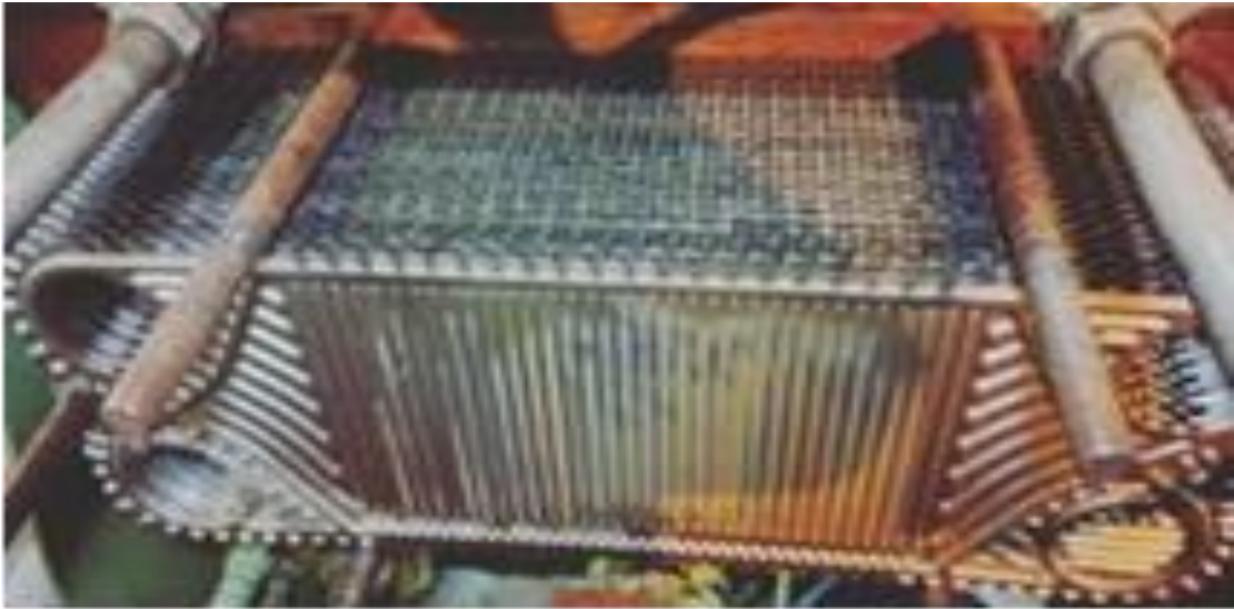
Lampiran 5 Kondisi plate Fresh Water Generator
