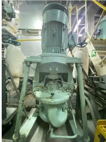
Gambar 2. 7 Pompa Sentrifugal Vertical
