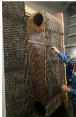
Gambar 2. 4 Heat Exchanger (Fresh Water Cooler) (Sumber: Dokumentasi Pribadi)
