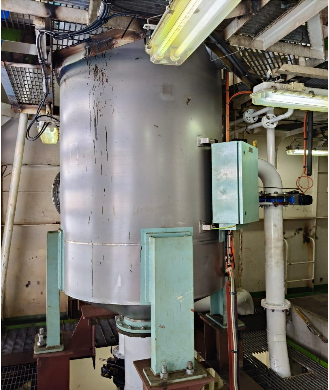
Lampiran 6. Scrubber Tower Inert Gas Generator
