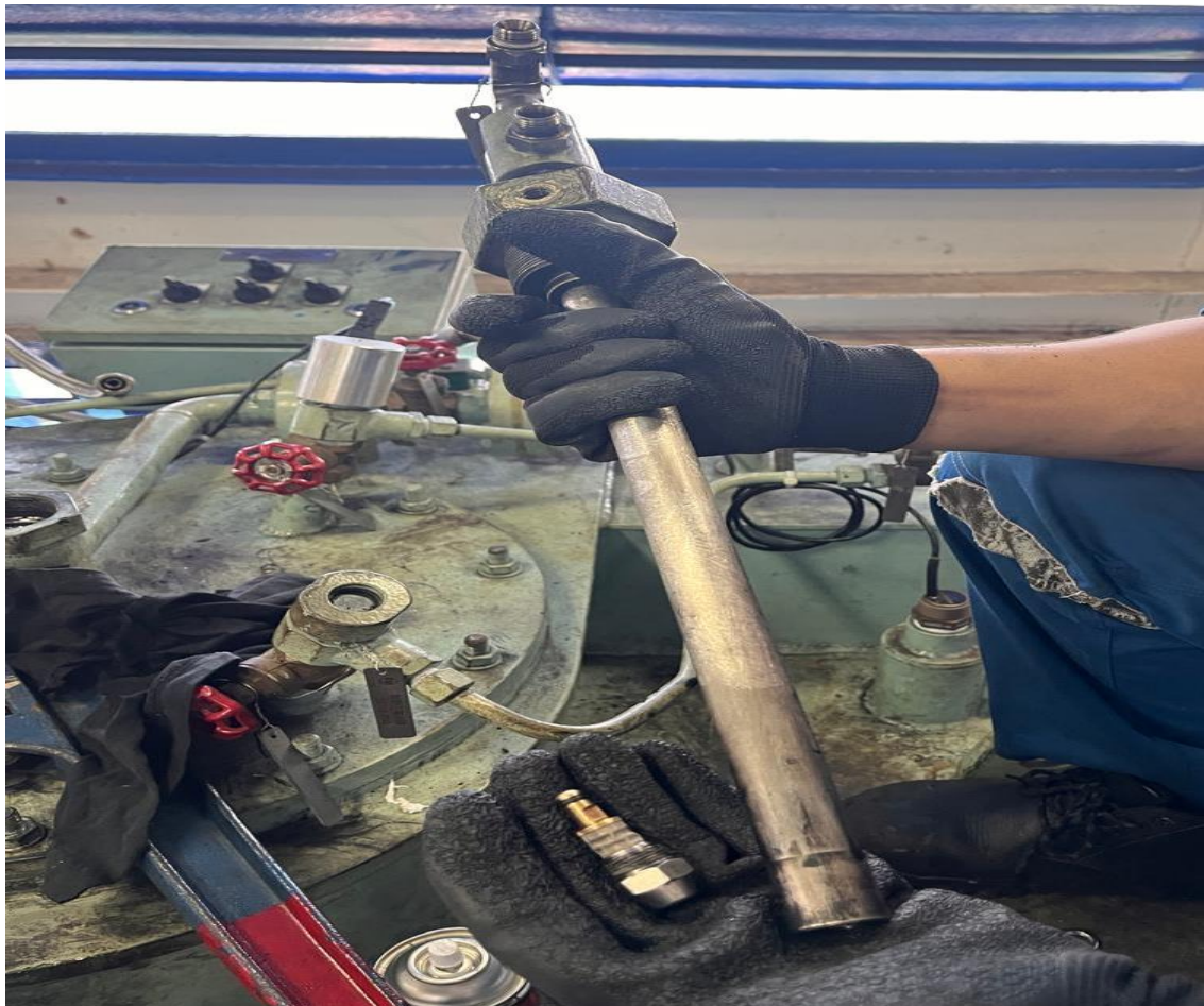
Lampiran 8. Kondisi Burner, Nozzle, Electrode Inert Gas Generator
