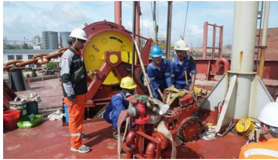
Gambar 2. 10 Maintenance windlass diatas kapal.
