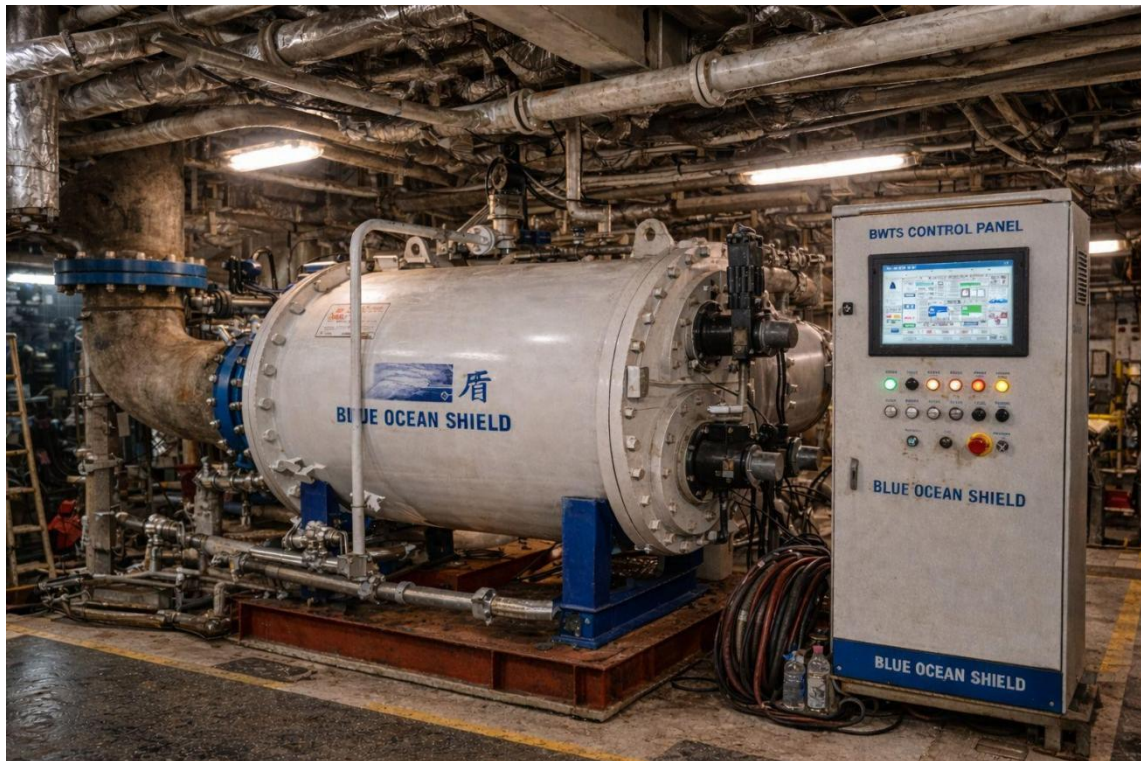
Lampiran 9 foto Ballast water treatment system
