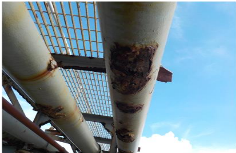
Gambar 4.1 kondisi Tank Cleaning Line MT. Ontari
